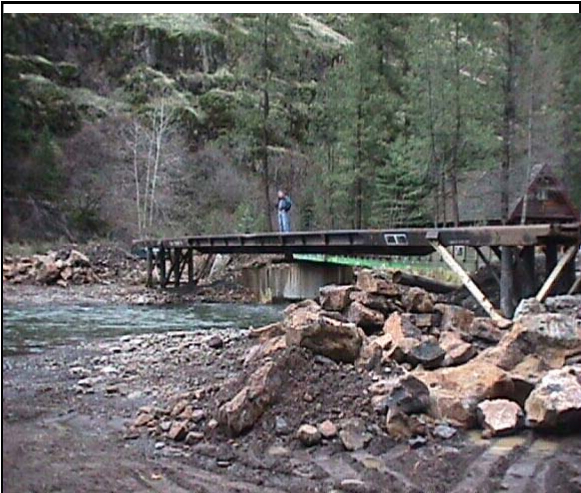
Figure J: 1997 Flood damage on Mill Creek (University of Oregon, Community Planning Workshop)
